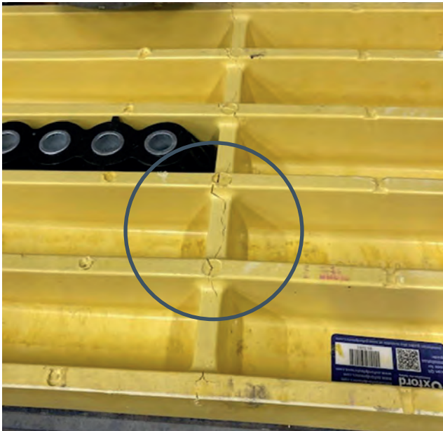
Crack along rib
